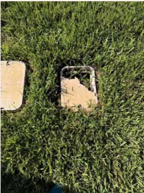
Broken Irrigation box at Village 3 Entracne
